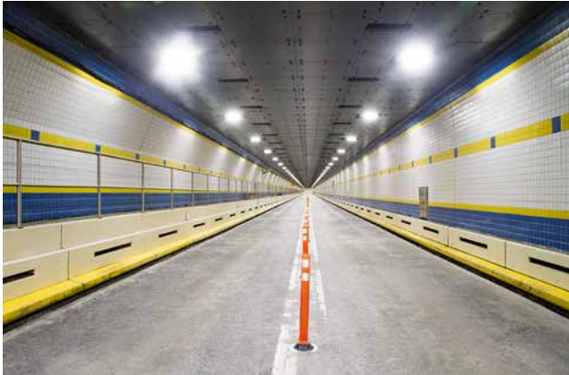
Even cleans the air in tunnels Hugh L. Carey Tunnel, New York, USA / Architect: HAKS, New York / Photo: Titus Kana
